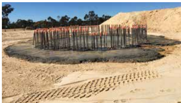
The blinding was poured to ensure returns from the Redbore 90 during piloting.
