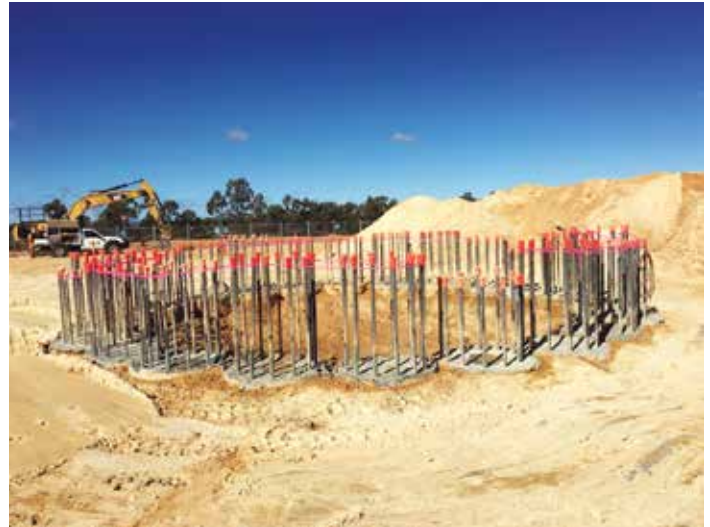
550m of piling completed in 11 days (22 x 25m each at 1050mm diameter.) All piles are within specifications, with no measurable vertical variance in any pile. Centre of piles was excavated to 4.0m from surface (RL 339.5) to enable a Client directed 40MPa concrete ring beam to be poured.
